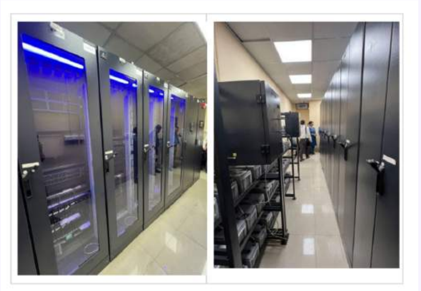
Figure 24: On Premise Data Centre Photos
