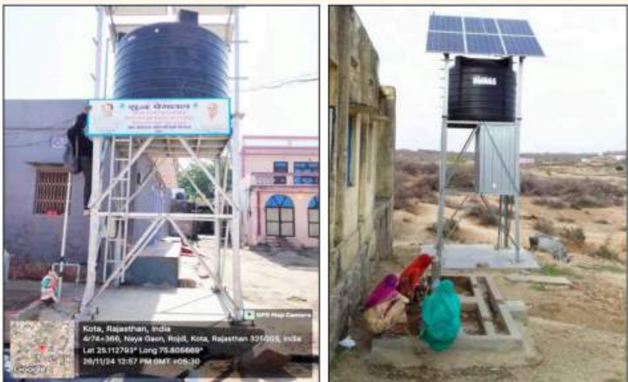
Figure 24: Solar Borewell System
