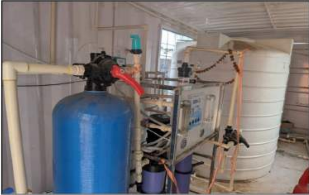
Figure 20: RO Unit Plant
