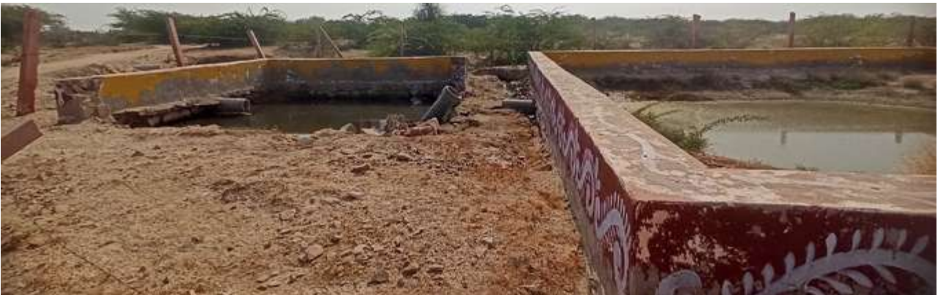
A portion of treatment system damaged due to heavy rains in Bhatinda Village, Luni Block, Jodhpur District,
