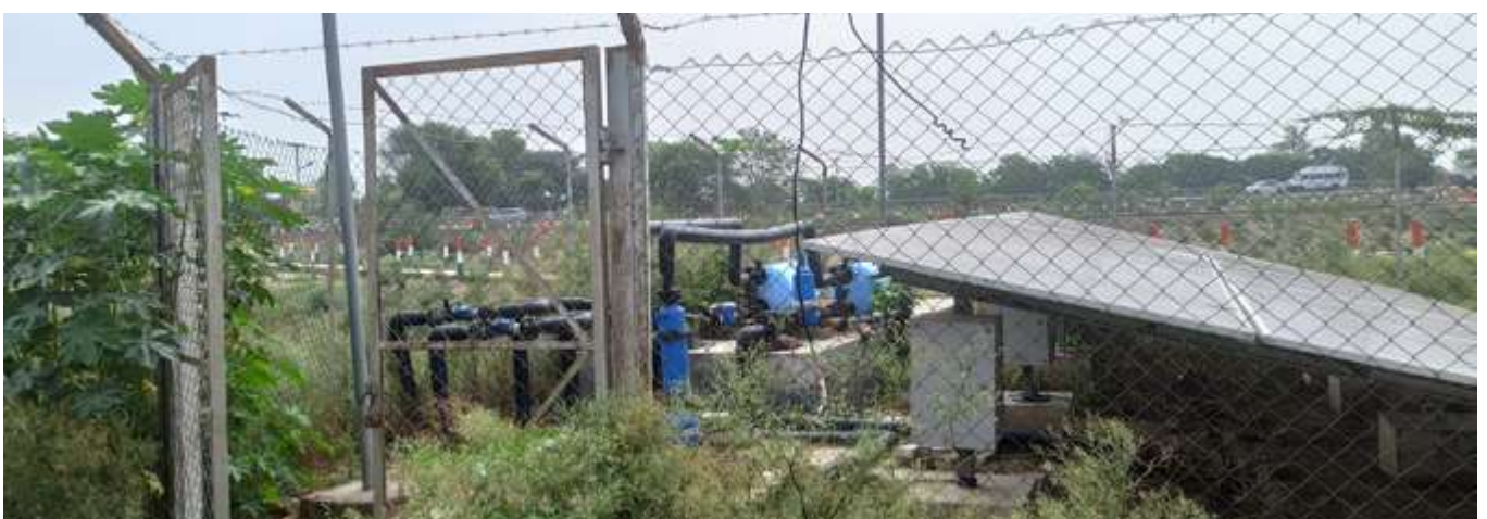
Solar powered pumping of treated greywater in Samana Bahu Village, Nilokheri Block, Karnal District, Haryana.
