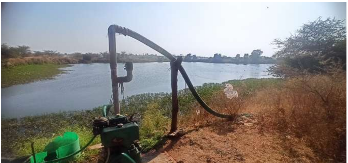
Untreated greywater being pumped for irrigation in Akesan Village, Palanpur Block, Banaskantha District, Gujarat.
