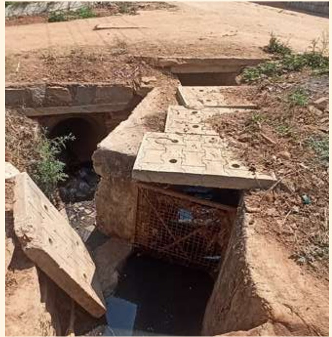
Separate diversion channels of stormwater and greywater in Muthur Village, Sidlaghatta Taluk, Chikkaballapur District, Karnataka.
