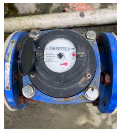
Bulk Flow Meters to track the volume of daily water supply
