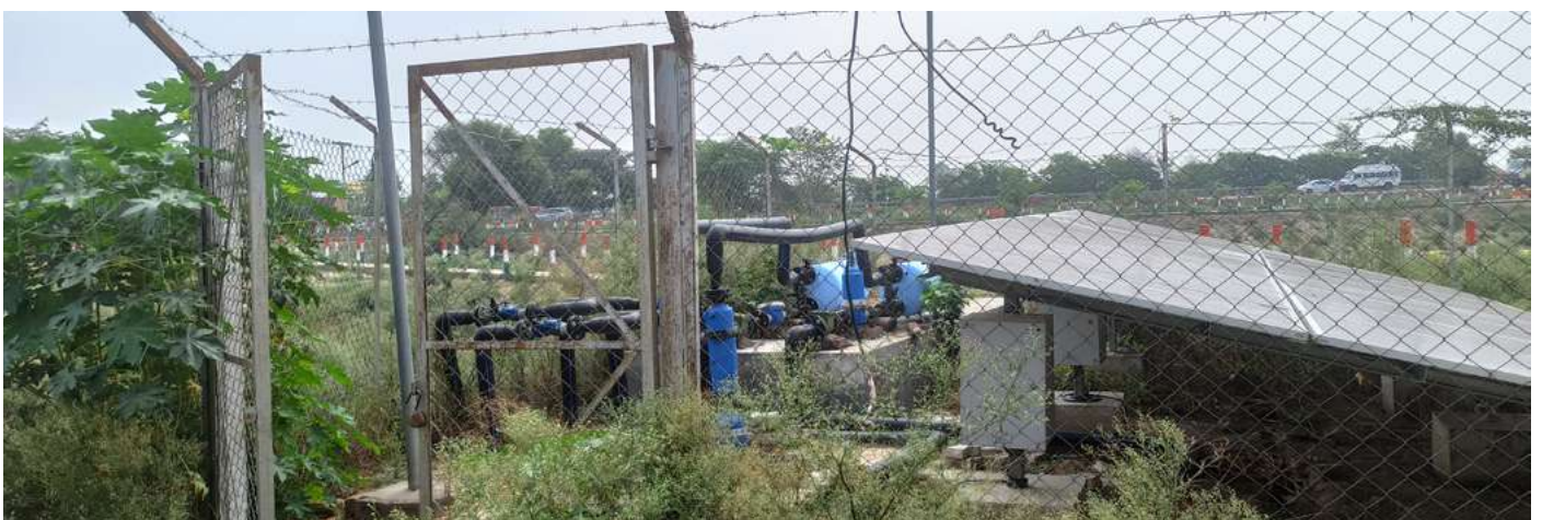
Solar powered pumping of treated greywater in Samana Bahu Village, Nilokheri Block, Karnal District, Haryana.
