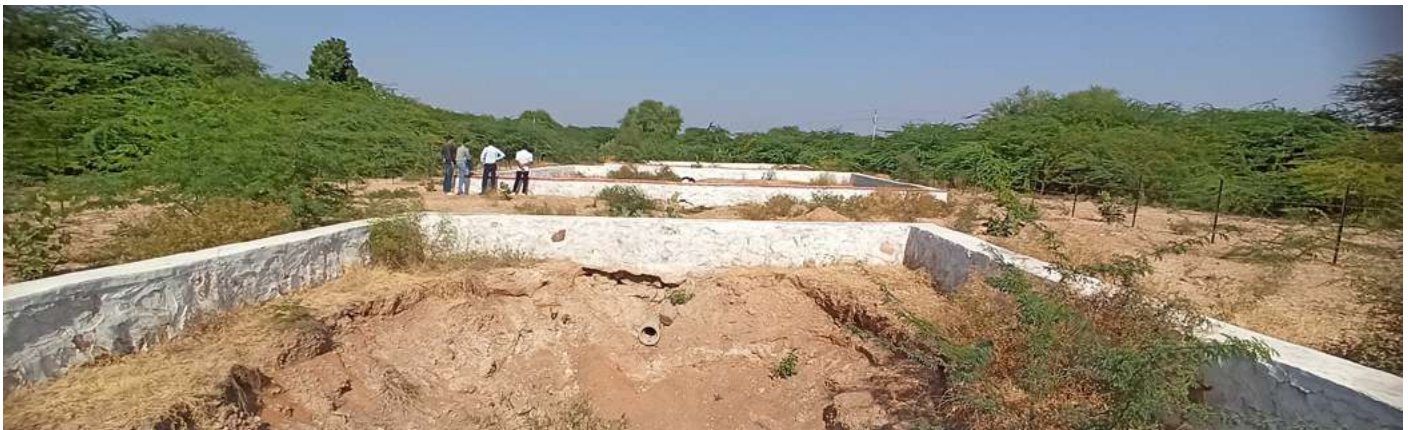
Treated greywater doesn't reach the Maturation Pond due to high evaporation rates in Sevaki Khurd village, Baori Block, Jodhpur District, Rajasthan.
