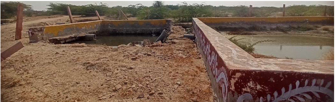
A portion of treatment system damaged due to heavy rains in Bhatinda Village, Luni Block, Jodhpur District, Rajasthan.
