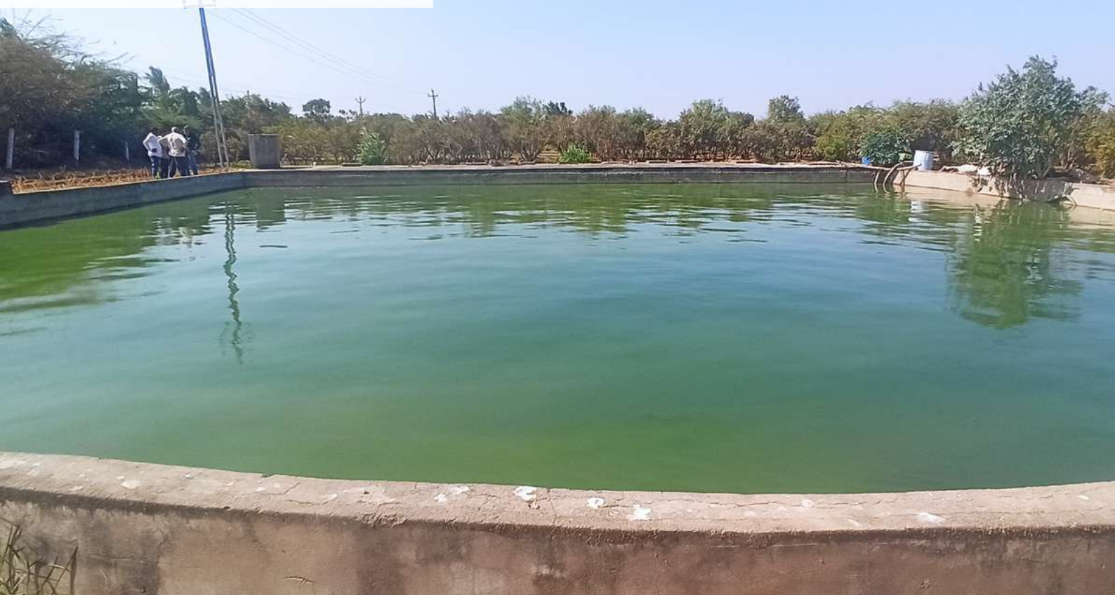
Maturation Pond of the DEWATS in Patia Village, Anjar Block, Kutch District, Gujarat.
