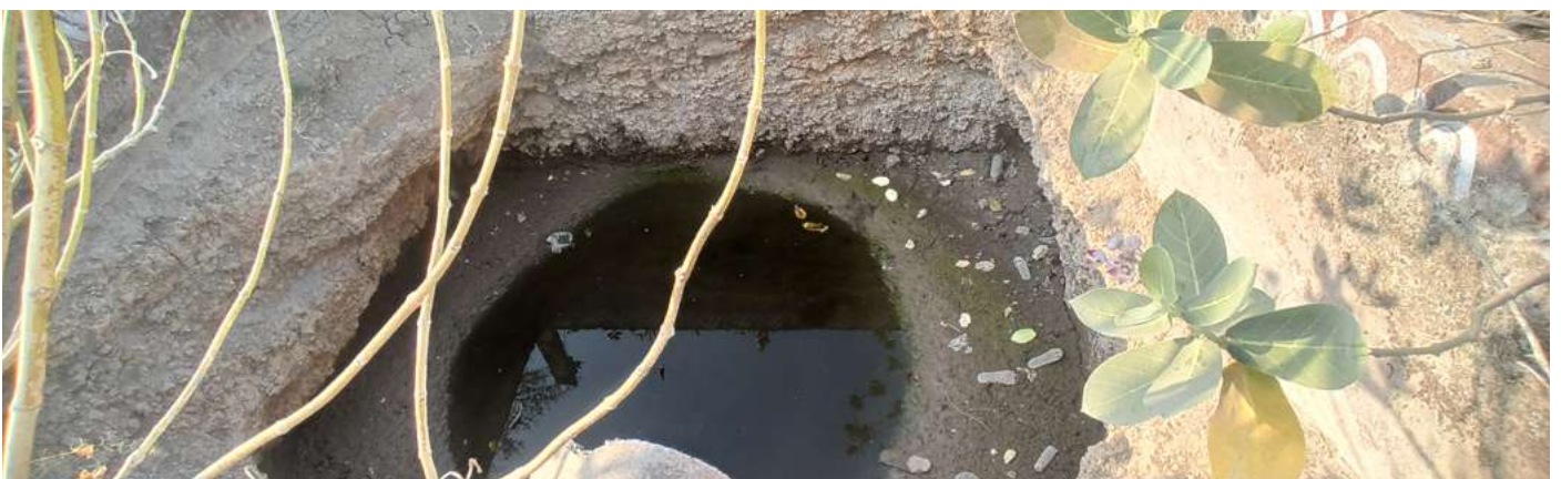
WSP showing little greywater collected in Daikara Village, Mandor Block, Jodhpur District, Rajasthan.
